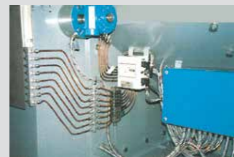
Centralized lubrication system
