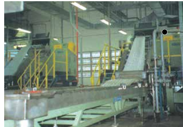
Cooling tank with air blade drying
